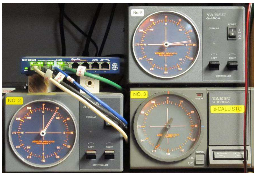
Figure 7 ~ G450-A controllers (upper-right and lower-left) and G800-SA controller, all modified with internal ERC modules and in active service. Only the G800-SA is shown tracking the Sun. Also seen in this picture is the 5-port Ethernet switch that handles LAN traffic for the equipment. (Images © 2015 W. Reeve)
