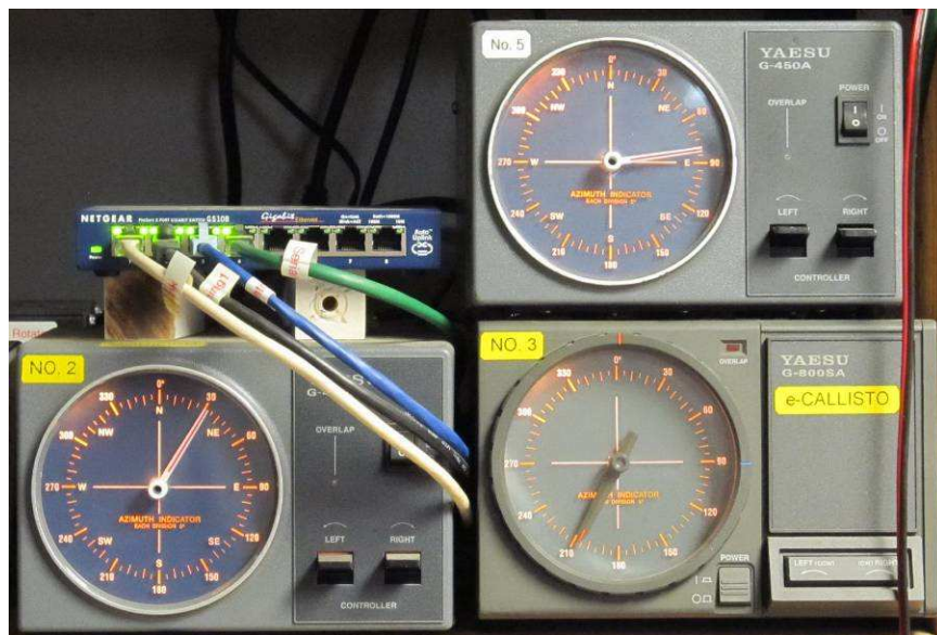
Figure 7 ~ G450-A controllers (upper-right and lower-left) and G800-SA controller, all modified with internal ERC modules and in active service. Only the G800-SA is shown tracking the Sun. Also seen in this picture is the 5-port Ethernet switch that handles LAN traffic for the equipment. (Images © 2015 W. Reeve)
