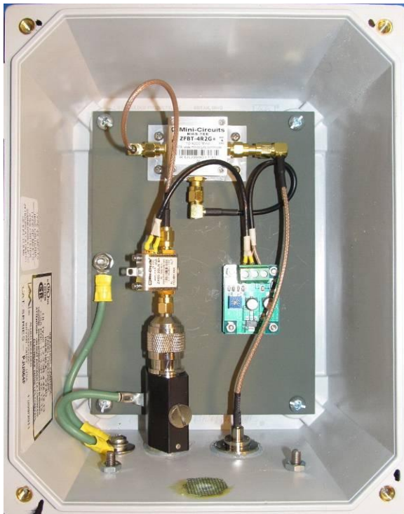
Figure 4 ~ Tower-mounted low noise amplifier. The TMA shown is a prototype, which used an adjustable internal voltage regulator (middle-right). The bias-tee is at top and the LNA module is middle-left. The black object at bottom-left is a lightning arrester.
