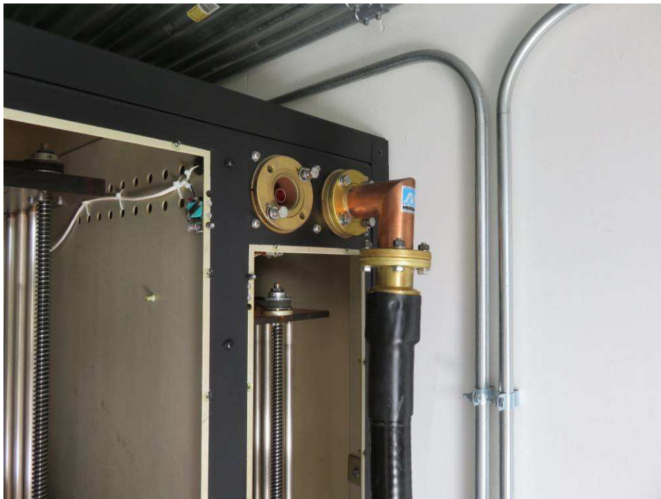
Figure 8 ~ Typical coaxial cable coupling at a transmitter. There are two connectors but only one is used. The coax appears to be 1-1/4 or 1-5/8 in air dielectric corrugated semi-flexible cable; however, I did not see any cable pressurization system manifolds or gauges so the cables may have a foamed polyethylene (PE) dielectric. The jack-screw tuning rods for the matching inductors (or capacitors) are visible in the open cabinet to the left of the cable. Image © 2016 W. Reeve
