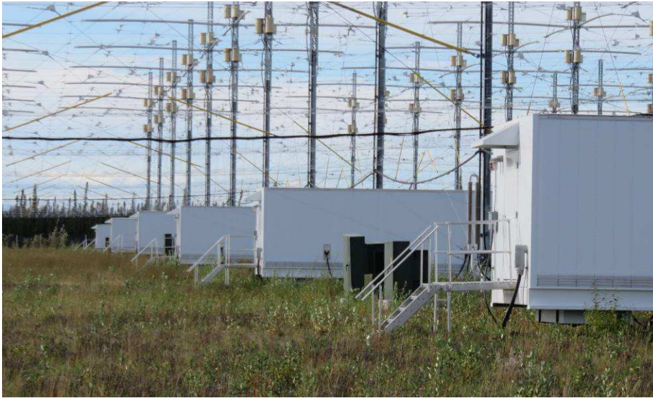
Figure 5 ~ The white transmitter enclosures appear to be modified shipping containers, 40 ft (12 m) long. The green enclosures near the center of this image are step-down power transformers and medium voltage (12.5 kV) sectionalizing terminals that serve two enclosures. Image © 2016 W. Reeve
