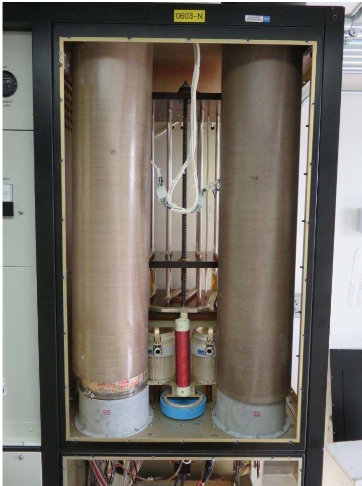
Figure 7 ~ Interior view of a transmitter cabinet. The HAARP transmitters use vacuum tube HPAs (high power amplifiers), and I believe this image shows two of the tubes with what appear to be cooling stacks. Image © 2016 W. Reeve
