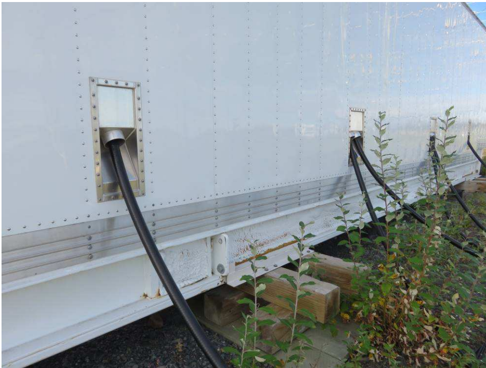
Figure 9 ~ Cable exits at a transmitter enclosure. The stacked timbers underneath the enclosures indicate the enclosures are free-floating and do not have thermal piles for foundation support. Image © 2016 W. Reeve
