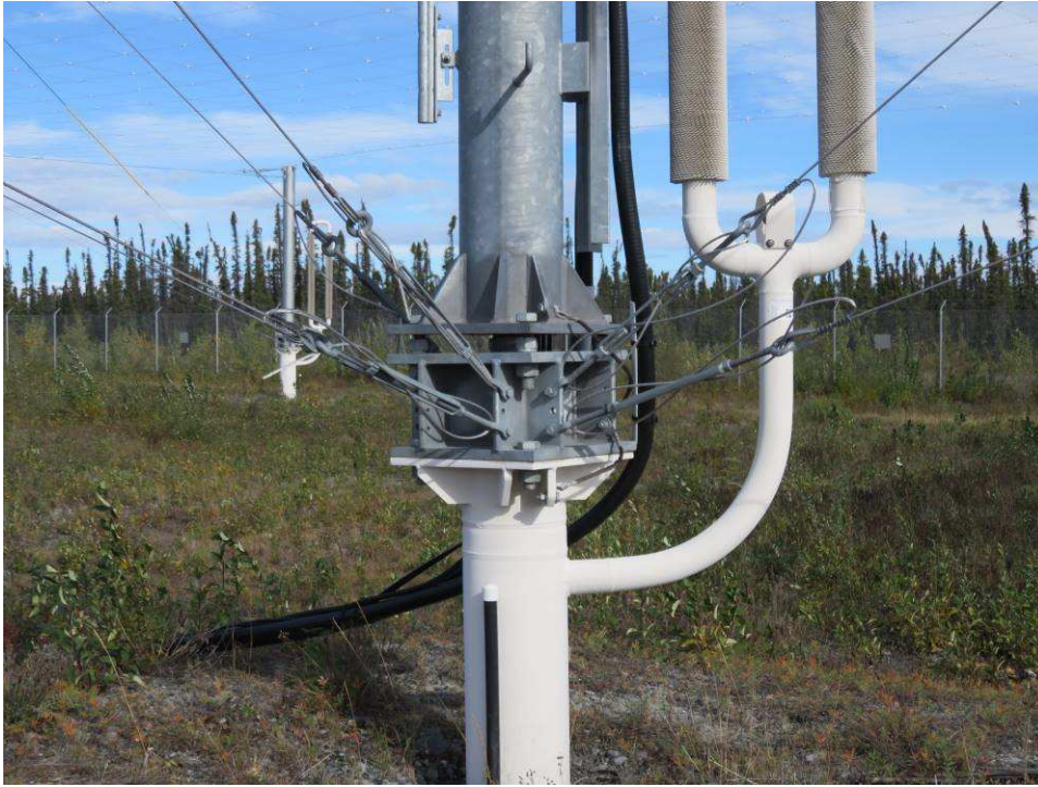
Figure 17 ~ Thermal piles are the white pipes shown here. The larger pipe provides mechanical support for each antenna support structure and keeps the ground frozen year-around. The galvanized steel tower base is mounted directly to the top of the pile and guy wires from adjacent towers connect to it for anchoring; the mechanical loads are symmetrical. The heat absorbing portion of the piles probably is buried a few tens of meters, and the heat is dissipated by the loop to the right. The black tubing behind the pile is the coaxial cable feeding the dipoles. Image © 2016 W. Reeve
